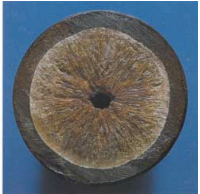
Galvanized pipe heavily scaled
