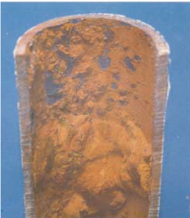
Galvanized pipe heavily corroded
