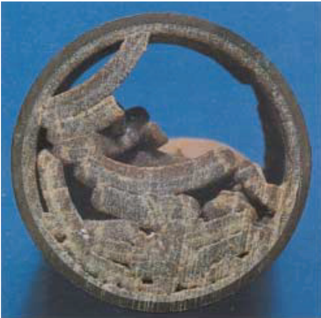
Copper pipe with scale plug
